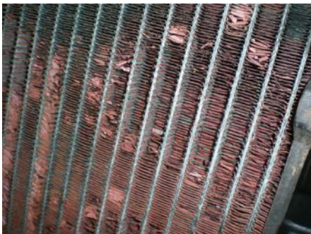
FIGURE 5-20 A heavily corroded radiator from a vehicle that was overheating. Visual inspection discovered that corrosion had eaten away many of cooling fins, yet did not leak. This radiator was replaced and it solved the overheating problem.
